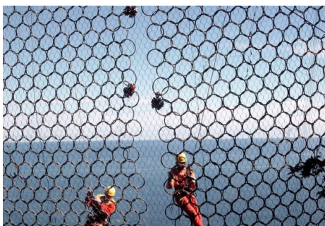
Protection system barriers
